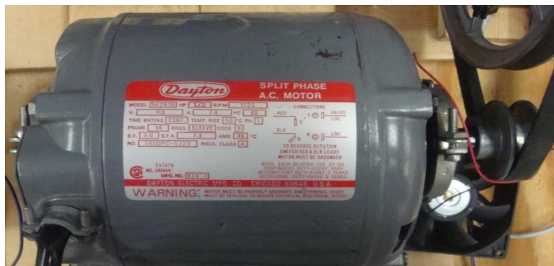
Figure 6.2 AC Motor connected coupled to shaft of Pump A
