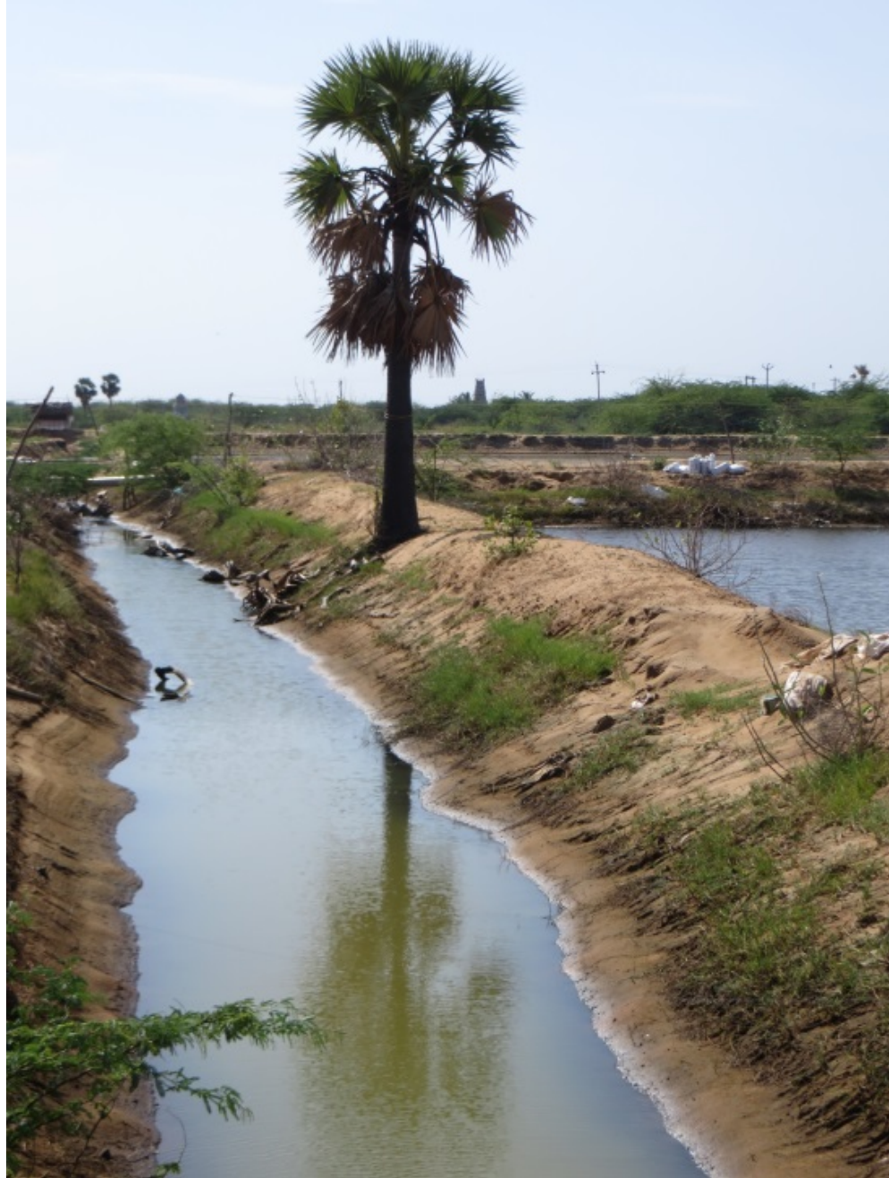
Figure 4. Water Seepage from Shrimp Pond
