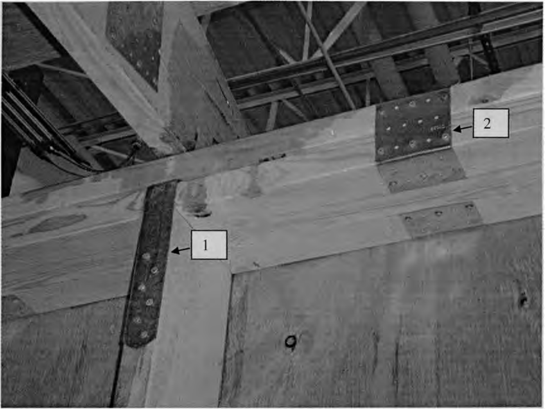
Figure 4.4 - (1) Strap holding the stud and the lower top plate together; and (2) U-shaped metal plates holding the upper and lower top plates together
