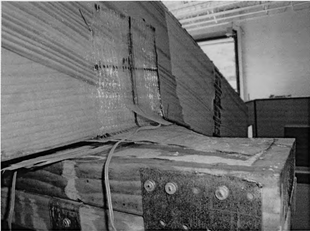
Figure 4.18 - Failure of FRP ties 19 and 20
