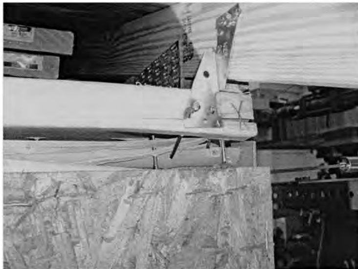
Figure 2.6 –Failed hurricane clip connection (NISTIR 6938 by Riley and Sadek, 2003)
