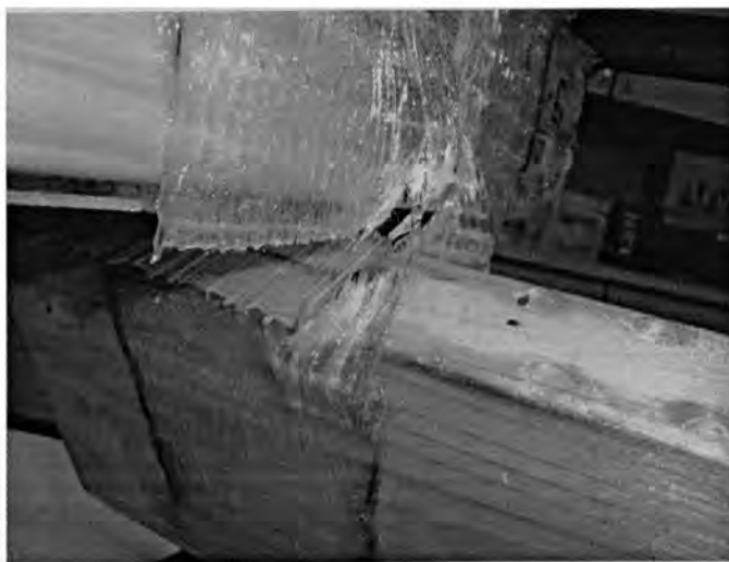
Figure 3.15 – Failure of FRP tie Configuration IV
