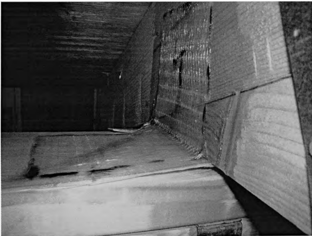
Figure 4.19 - Failure of FRP ties 7 and 8 and separation of wood fibers
