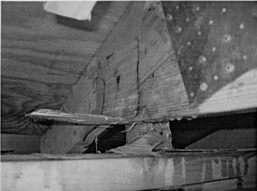
Figure 4.16 - Complete failure of FRP ties 13 and 14 at 23,659 lbs
