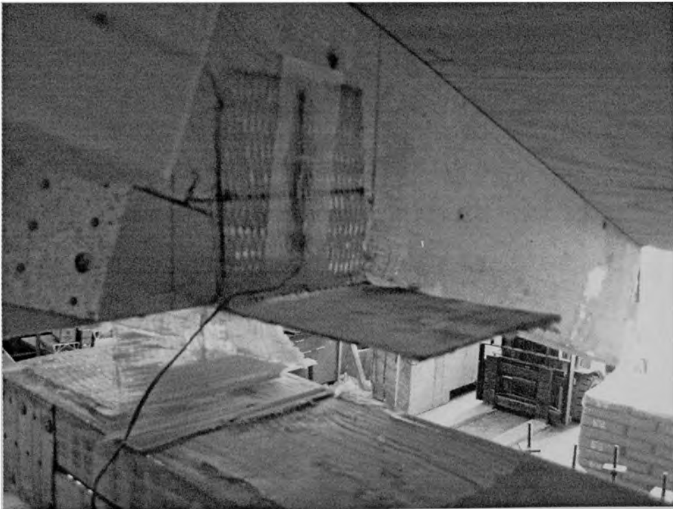
Figure 4.17 - Failure of FRP ties 11 and 12
