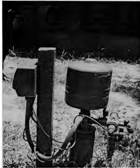
Figure 8 - Discharge and suction wells; green painting as an aesthetic idea.
