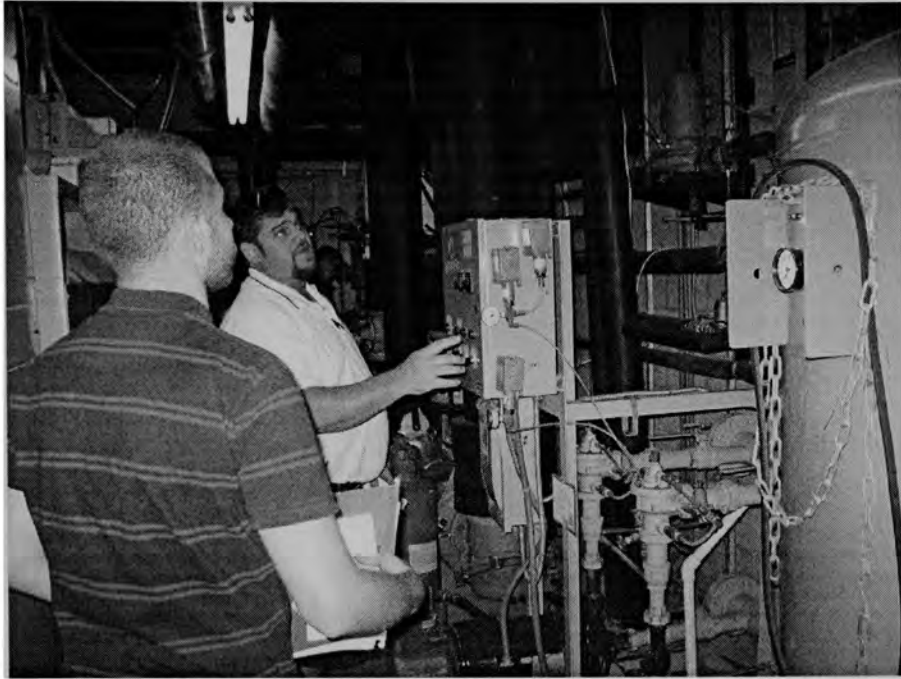
Figure 14 - Springhill Suites Mechanical room
