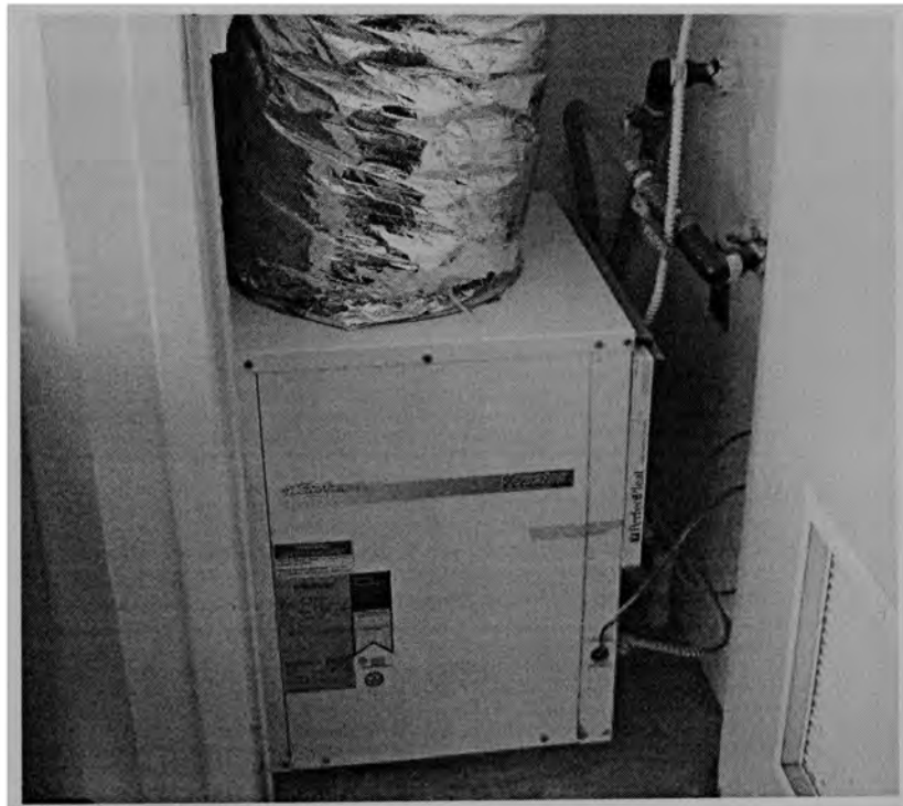
Figure 13 - Springhill Suites Indoor heat pump unit
