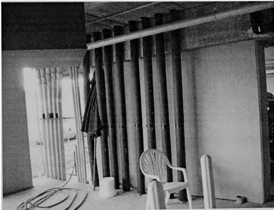
Figure 15 - Springhill Suites Supply and return pipes
