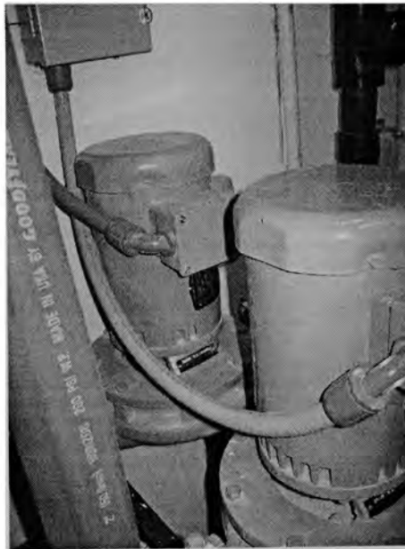
Figure 22 - Rodney Rich building Main loop pumps
