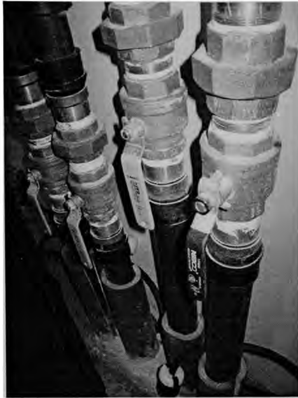
Figure 23 - Rodney Rich building-Supply and return pipes
