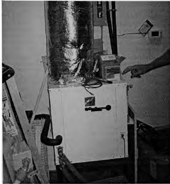
Figure 21 - Rodney Rich building 1 ton unit
