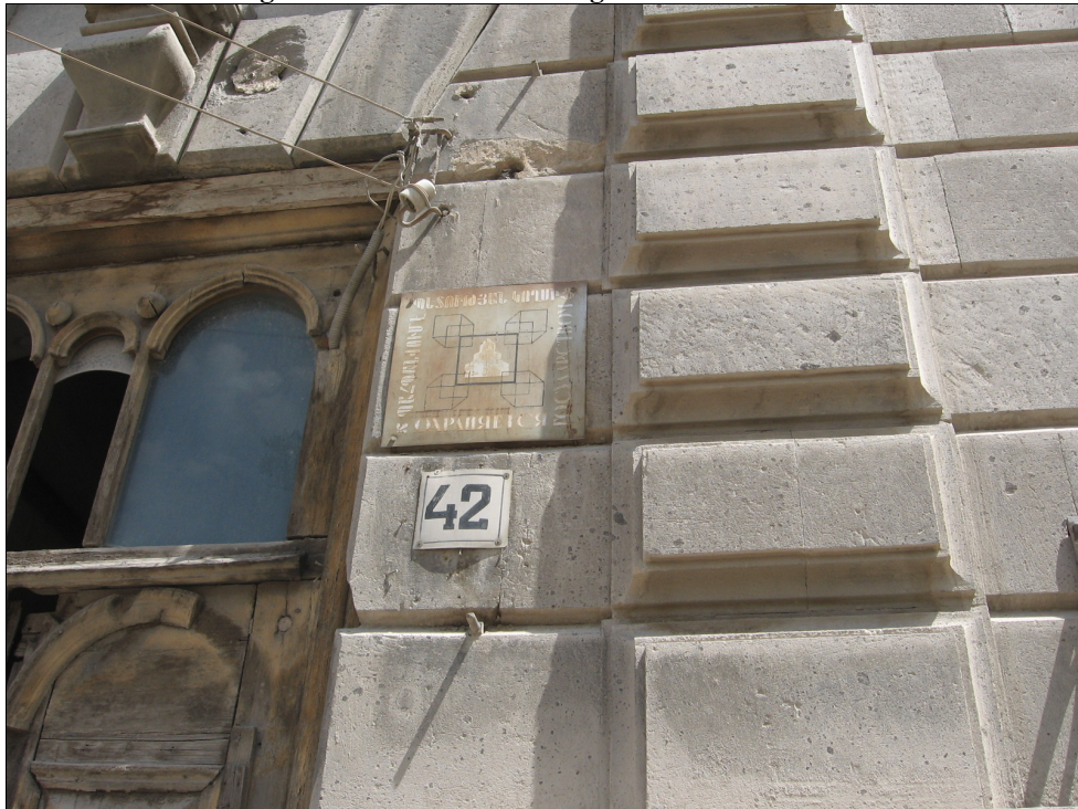
Figure 4.4: A "black building" on Buzand Street. The plaque reads "protected by the government" and designates protection under Soviet law.
