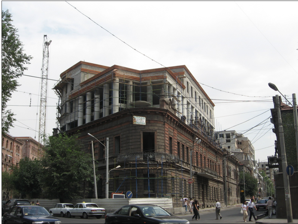
Figure 4.7: A "black building" on Hanrapetutyán Street. This building is being restored on site.
