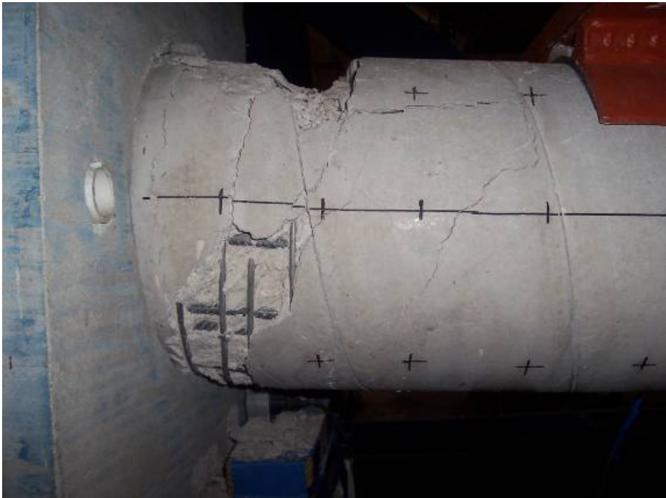
Figure 4.12 East View of Final Cracking Pattern Close to Footing in Specimen RC
