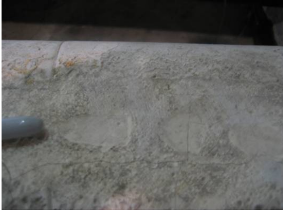
Figure 3.15 Small Pockets of Concrete Void along the Top of Specimen RC
