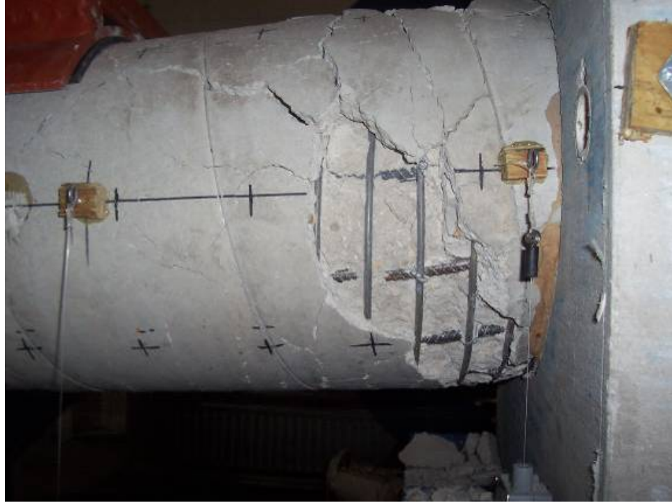
Figure 4.13 West View of Final Cracking Pattern Close to Footing in Specimen RC
