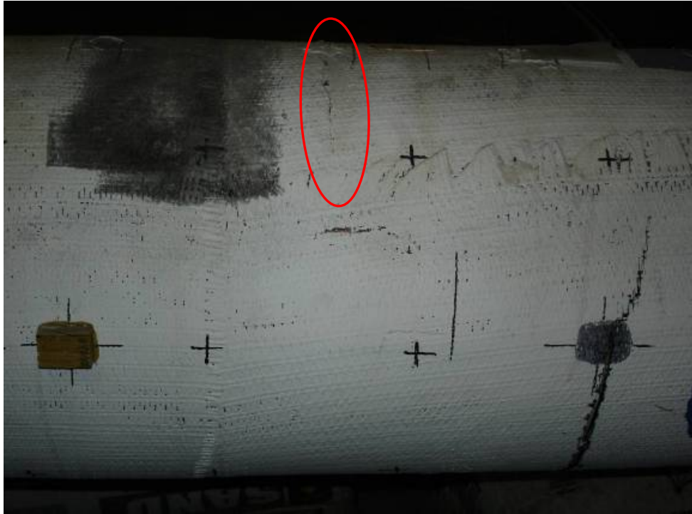
Figure 4.25 Crumpling Crack in Specimen SC (West View)
