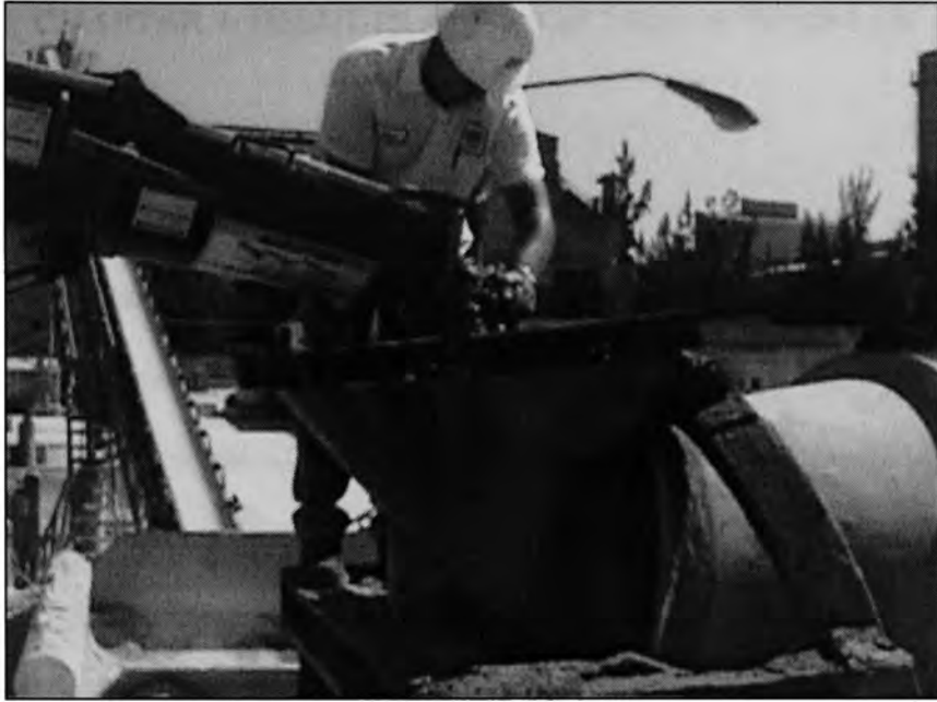
Figure 3.7 Concrete Cement Lump Retrieval
