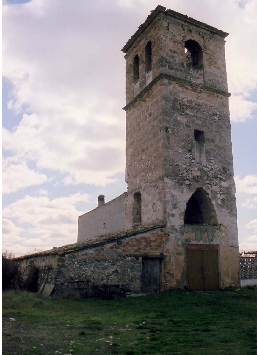
Figure 35. Bell tower. Site of Augustinian monastery of San Blas, Villaviciosa del Tajuña.
