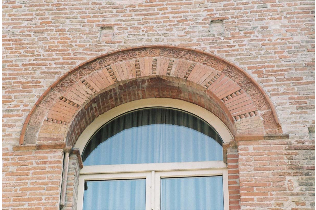
Figure 74. Terracotta decoration on west window of Great Hall. West front. Palace, Cesena.
