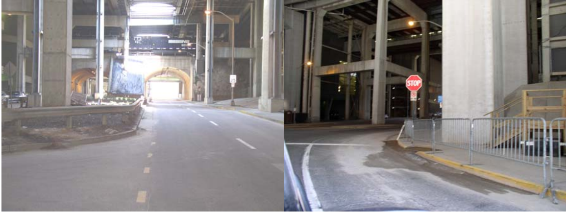
Figure 85: Location G is a very complex steel structure with many tunnels and ramps.
