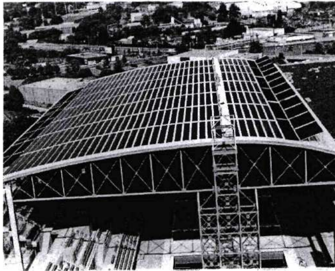
Figure 4. Aerial view of the Georgia Tech Aquatic Center (GTAC) rooftop PV array, showing the roof curvature.
