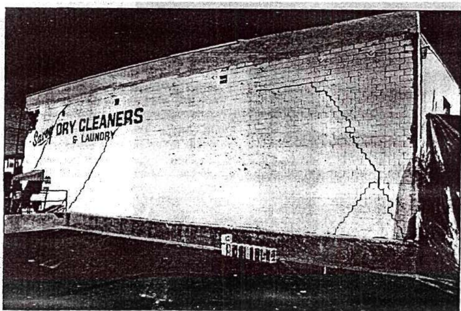
Figure 2.35. Damage sustained prior to retrofit with FRP overlays (taken from
