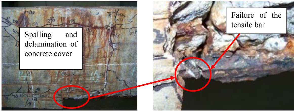
(a) Failure of the corroded beam B2C13 due to tensile bar rupture
