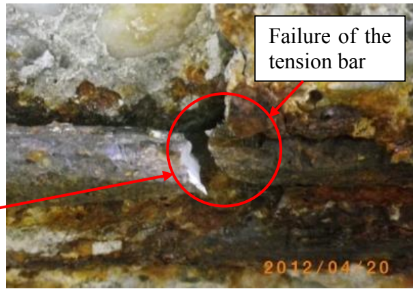
(c) Failure of tension bar of B2C13-2
