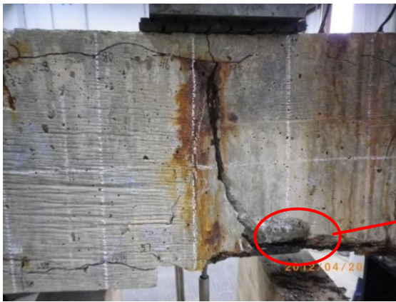
(b) Failure of corroded beam B2C13-2
