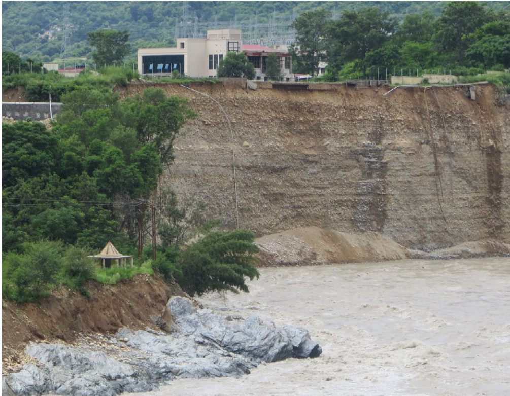
Figure 4: Erosion of muck disposal site at Srinagar Dam, after the flood of June 2013.
