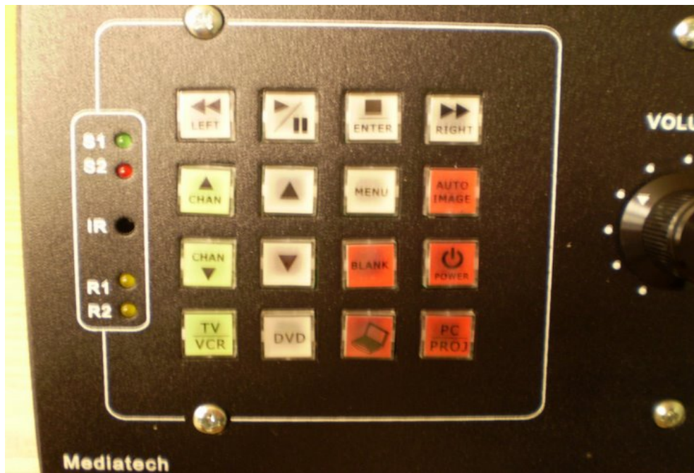
Equipment Rack Control Panel: Medatech 52
