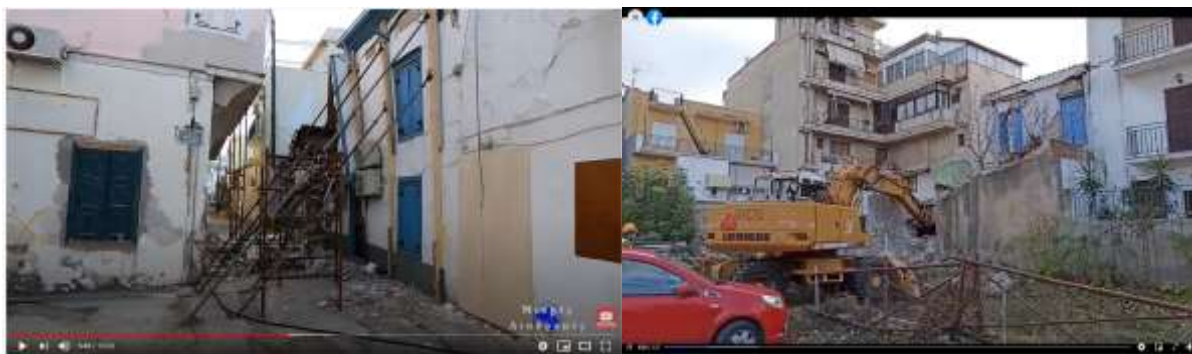
Figure 122: Shoring of near collapse buildings (“Mikres diadromes” you tube channel) and demolition of dangerous buildings (“Agakliazo ti Samo” facebook page)
