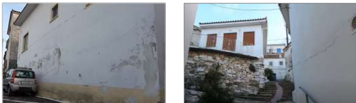
Figure 64: Damage in masonry buildings in Samos with horizontal cracks at floor level due to sliding (Photo credits to "Mikres diadromes" youtube channel)
