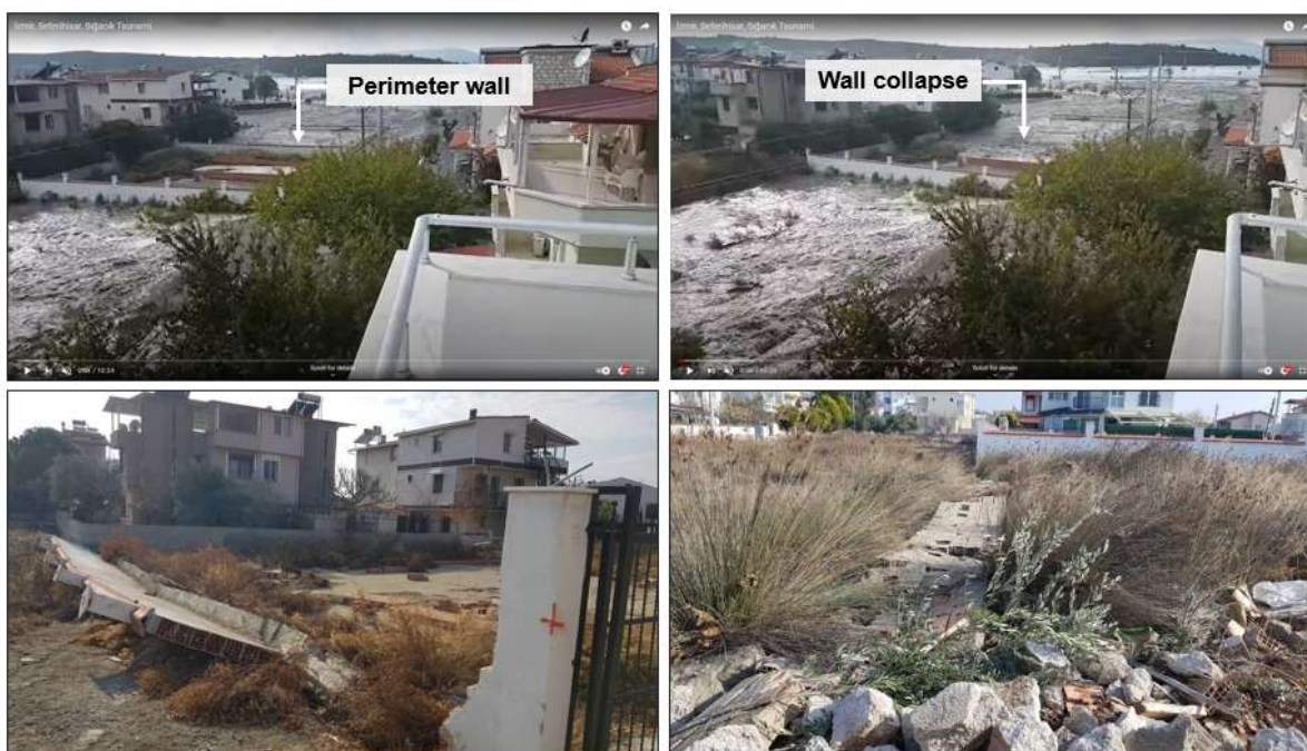
Figure 106: Perimeter wall overturning due to tsunami hydrodynamic effects in Sığacık (coordinates: 38.1982930, 26.7902697). Video frames (on top) from YouTube video: https://youtu.be/n93puRYKhs0
