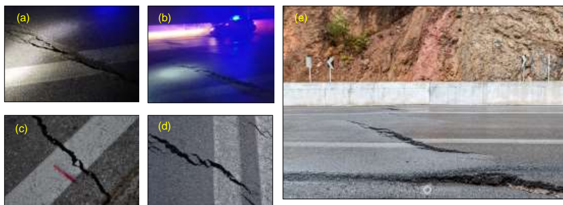
Figure 35: Road cracks observed in the area of (a) Vathy-Karlovasi road (Vadaloukas et al., 2020), (b, c) Agios Nikolaos (Lekkas et al. 2020), and (d) the main road Vathy-Karlovasi close to Karlovasi (photo taken by Manolis Thralvalos)
