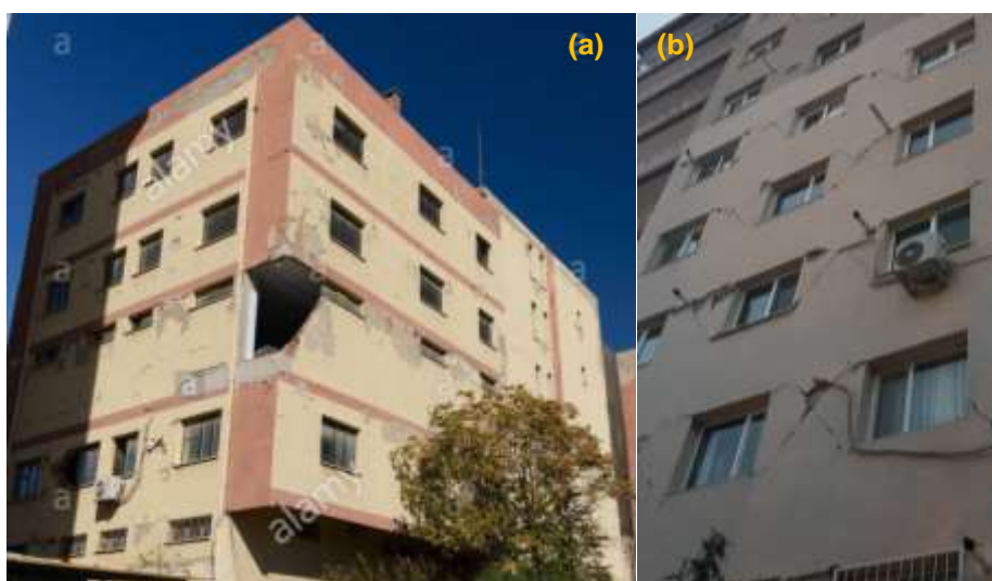
Figure 82: Infill walls damage in RC frames: (a) out of plane (Arda Savaşcıoğulları / Alamy Stock Photo) and (b) in-plane failure
