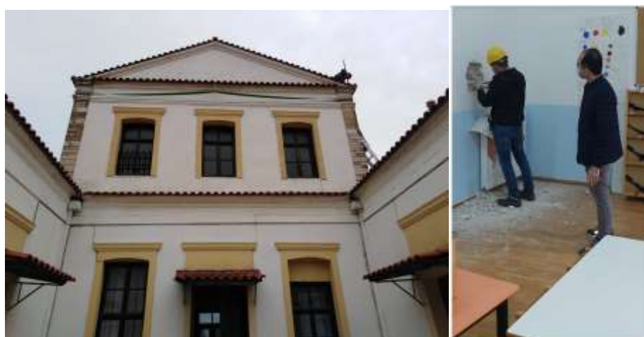
Figure 123: Primary school of Mitilinioi, confinement of the walls with external straps (left); repair works at Agios Konstantinos Primary School, so that their function can be resumed (Municipality of Eastern Samos Facebook page, 16.01.20)
