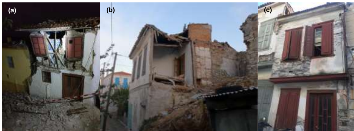
Figure 94: Examples to damage in hımsı structures
