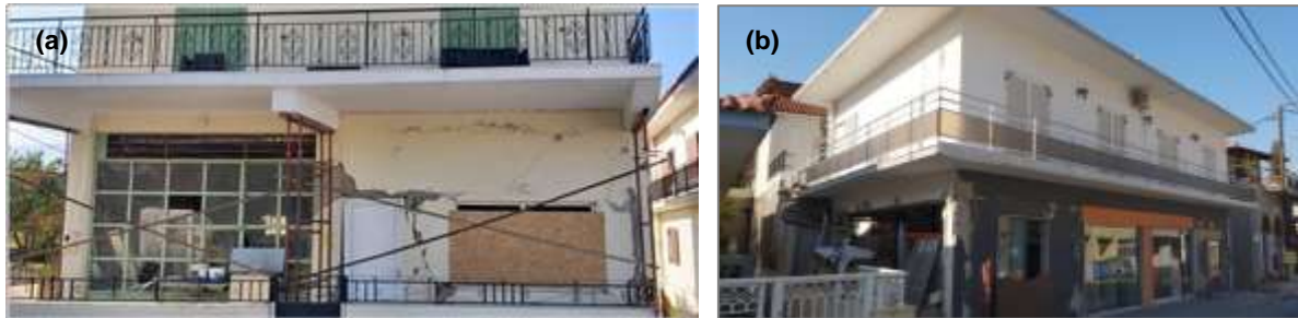
Figure 60: Damage to infill walls in two RC buildings in Samos: (a) in plane and (b) out of plane failure
