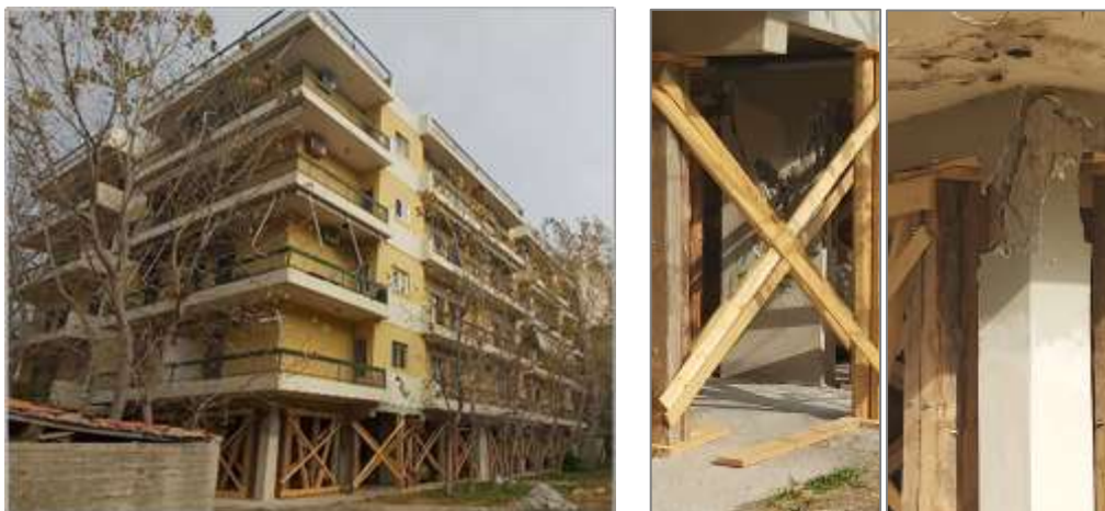
Figure 61: Five-storey building with soft first storey (pilotis) failure at the ground level in Karlovasi (Samos)
