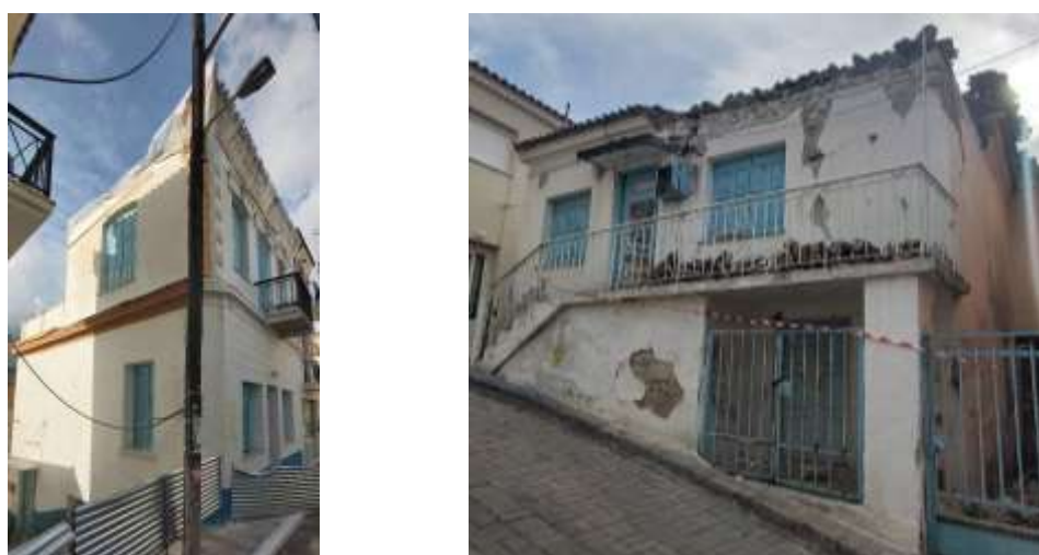
Figure 65: Roof damage to masonry buildings in Samos.
