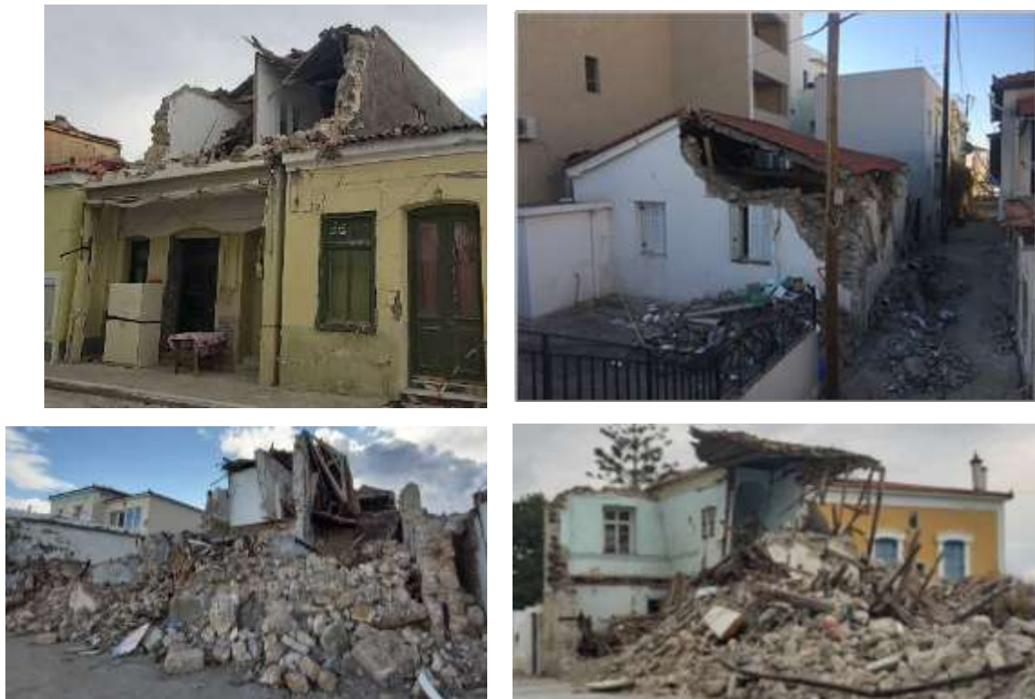
Figure 68: Partially and totally collapsed buildings in rural localities and Samos town.
