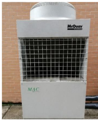
(a) Air-source heat pump
