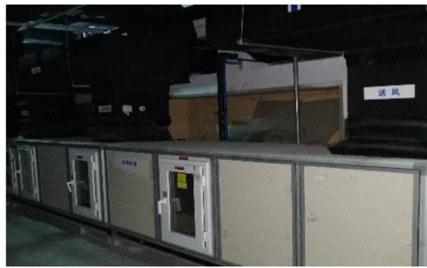
(b) Air-handling unit
