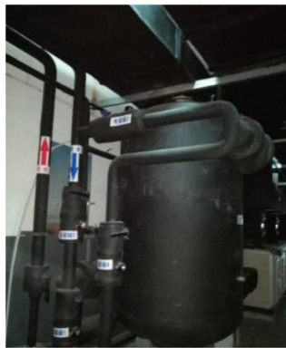
(c) Energy storage tank
