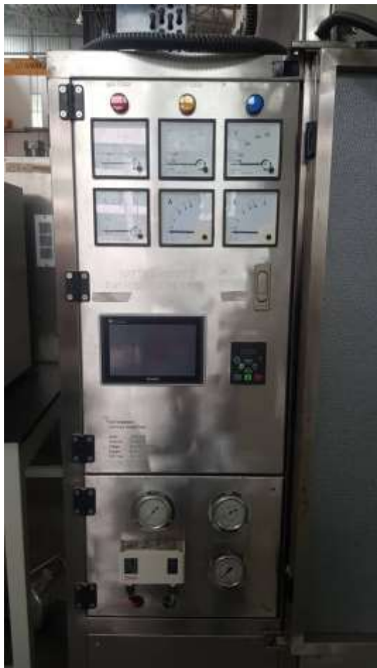
Figure B1 Control panel for Heat pump dryer
