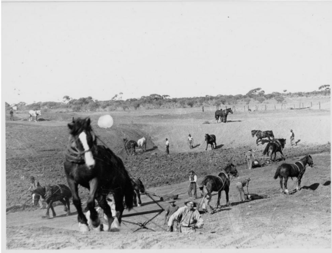
Figure 13: Railway Dam under construction in 1917. Establishing permanent water supplies was an essential part of railway construction. Source: State Library of Western Australia 209894PD.
