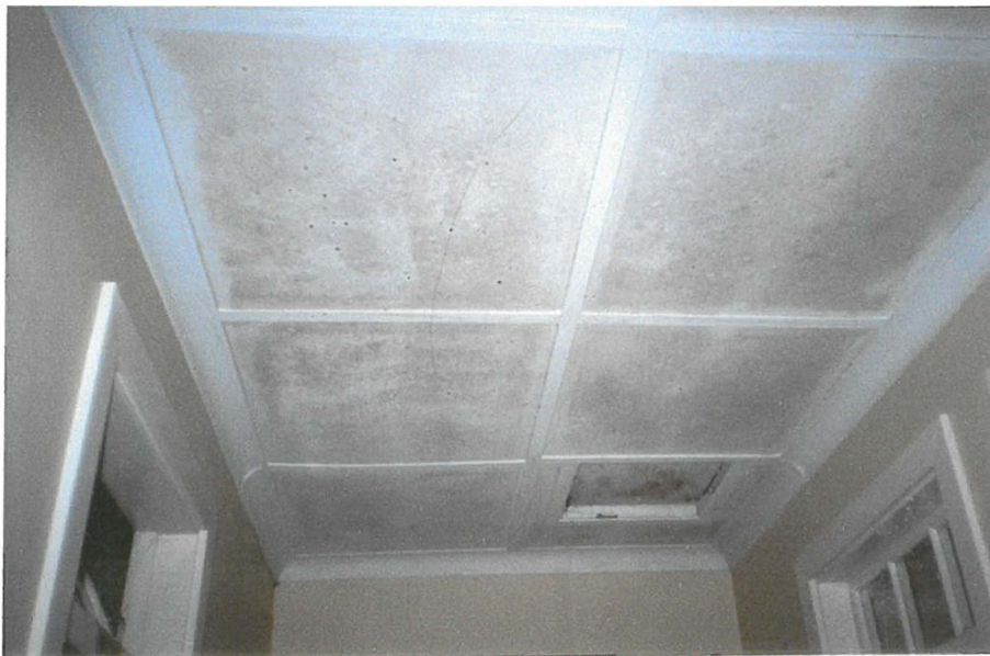
Figure 4. Mouldy ceiling in a hospital ward.
