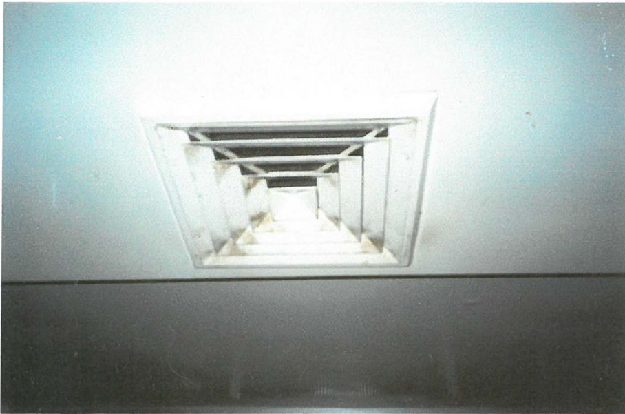
Figure 5. Mouldy ward office air conditioner outlet and ceiling
