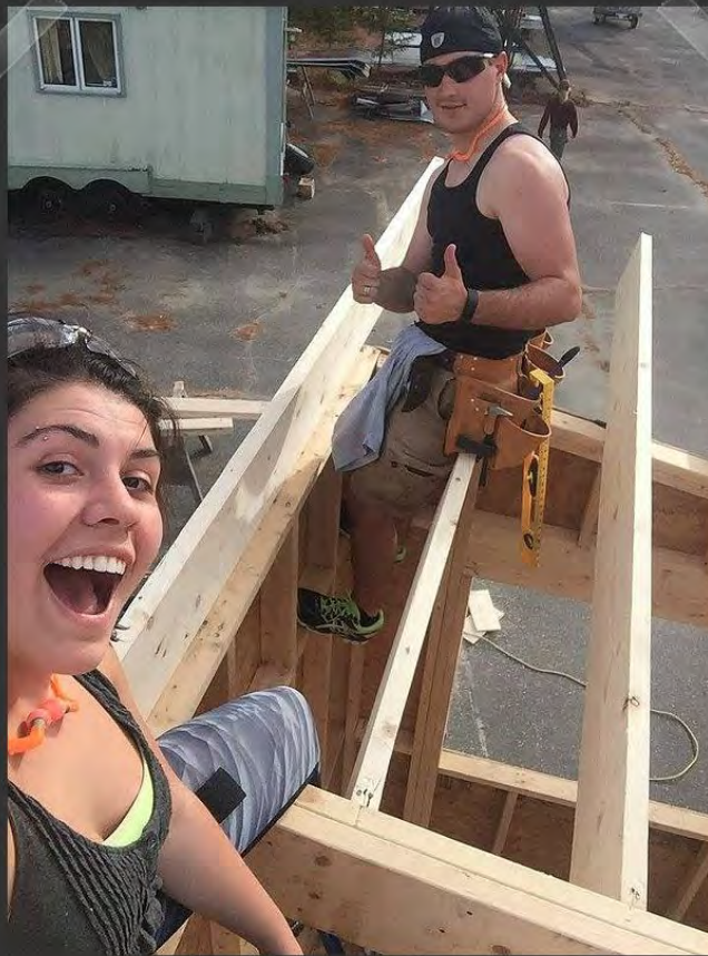
Nathan and Gwen, claiming their title as Roof King & Queen for being the most dedicated people to work on the roof.
