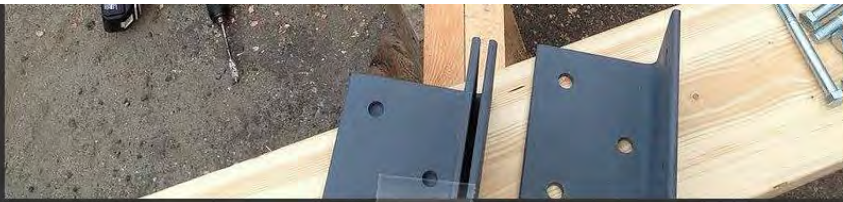
Installing corner brackets in between the floor joists and on each corner of the floor-packs.
