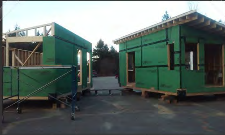
Library (right) is fully sheathed, including roof. Residence (left) is still in the sheating process. Mudroom will go in between the two.
