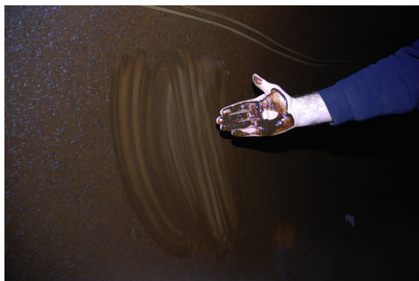
Fig. 2. Photograph from inside trunk main showing material adhesion across all boundary surfaces.
