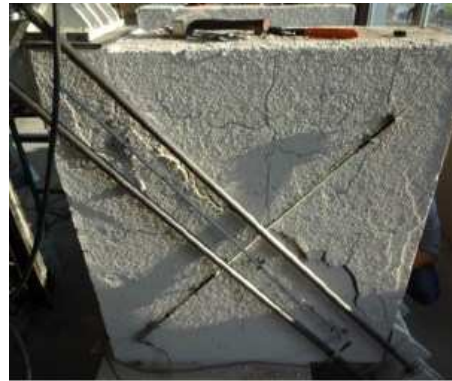
Figure 9 – Failure mode for panel reinforced with mortar type RO
