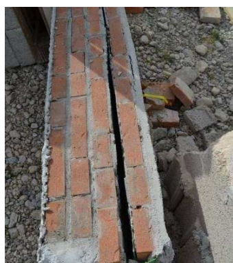
Figure 25 – Detail of a brick masonry ring beam after failure
