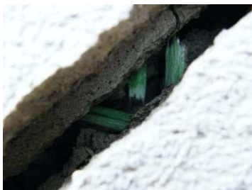
Figure 10 – Detail of the GFRP mesh after cracking
