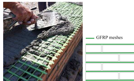
Figure 21 – Clay brick FRCM ring beam
