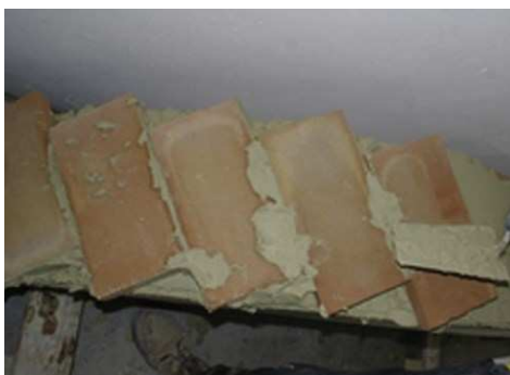
Figure 14 – Detail of unreinforced arch
