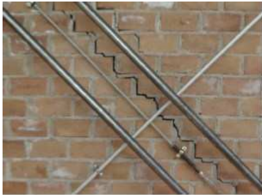
Figure 8 – Failure mode for unreinforced panel
