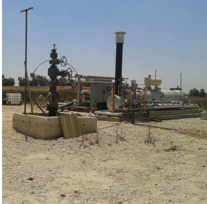
Figure 20. Connection to the injection well.
