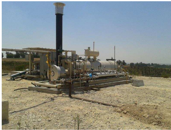
Figure 18. The heat exchanger.
