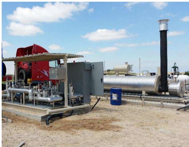
Figure 19. Pump skid during commissioning.
