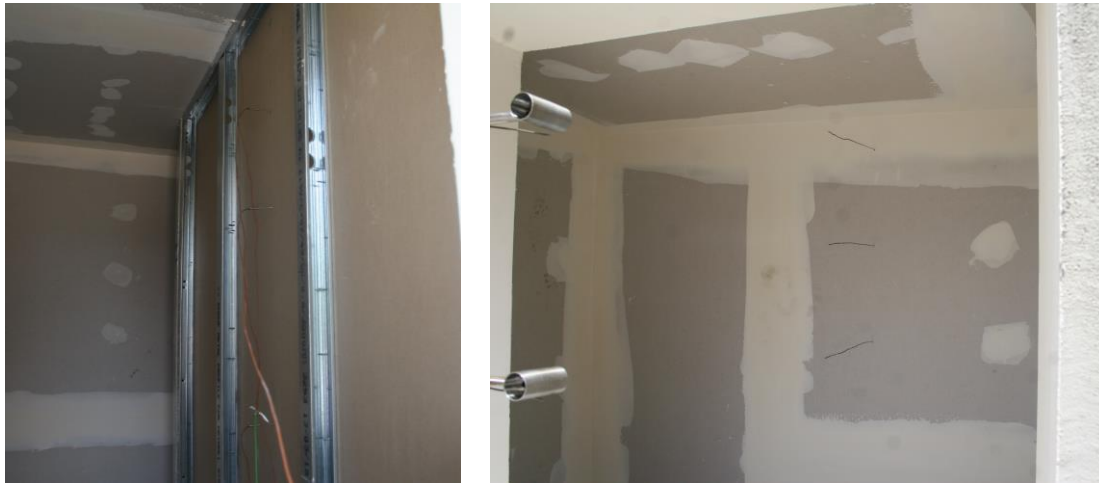
Figure 6-11. Positioning of the thermocouples at the interior of the fire compartment, indicative picture of the non-exposed side of the south compartment wall (left) and their positioning at the geometrical center of the room (right).
