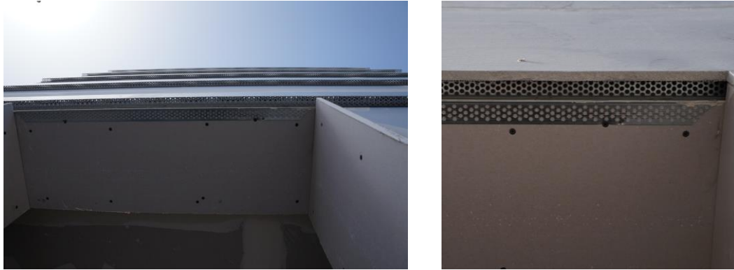
Figure 6-7. Construction details of the upper side of the window opening before (left) and after (right) the positioning of the cement board.
