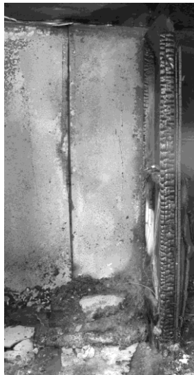
Figure C-3. Post-fire photograph of the western timber frame and the wood-based panel protected timber frame wall assemblies.
