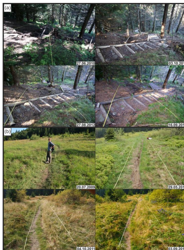
Figure 5. (a) Case study C – an example of a trail which has been degraded and repaired. The old course of the trail is marked by yellow survey tapes. After the event, new, less steep course was designed and wooden and stones steps were installed. Note that erosional processes are still active within the old route. (b) Case study D – an example of trail which was degraded and left for natural recovery. Note that before the intense rainfall event, the trail was undamaged and very narrow. In May 2010, an erosional rill developed and as a result of this, visitors created a new path (visible since 2011). During the recovery period, the grass had partly overgrown the rill; however, geomorphological processes were still active.
