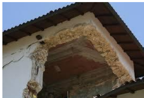
Figure 2. Example of an out-of-plane collapse due to poor connection between the RC ring beam and the underlying masonry.
