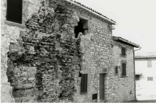
Figure 1. Example of separation between two leaves of masonry due to seismic action.
