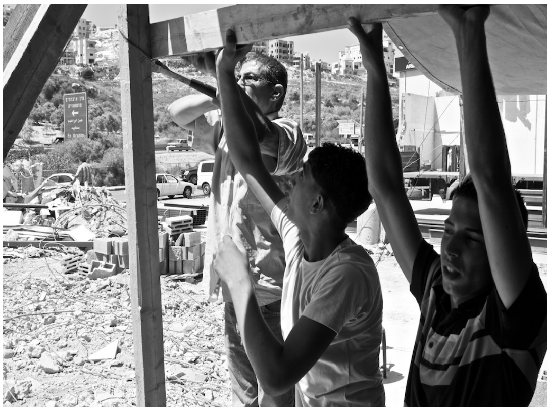
Figure 29: Rebuilding the fruit and vegetables store which was demolished in the market area
