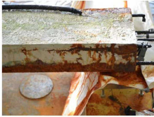
Fig. 4. Longitudinal cracks observed during corrosion
