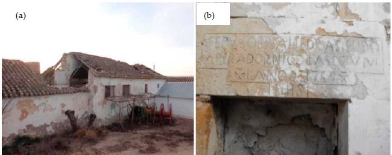
Figure 12. (a) State of the roof, partially torn down, of the “Lagar de Las Monjas” in Montilla (Córdoba) [43]; (b) lintelled stone signed by the implementer in the year 1769 in the mill of the “Lagar de las Monjas” [43].
