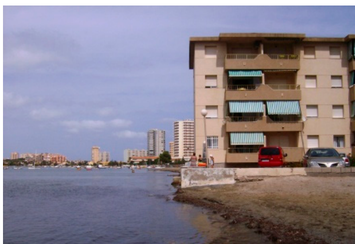
Figure 7. Extreme retraction in numerous beaches on the Mar Menor side of La Manga that currently reach the foundations of the houses.
