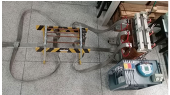
FIGURE 15. Upper view of the test set up for voltage application of bus bar laid on supports.
