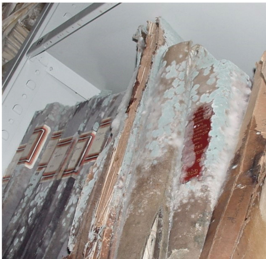
Figure 1. Fungal outbreak as a result of leaking water from the roof of a depository room (AHU-DGLAB, Portugal, 2005).
