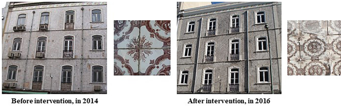
Figure 5. Illustrative example of a major intervention in which the initial condition was not restored.
