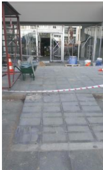
a) Blocked access to classrooms building.
