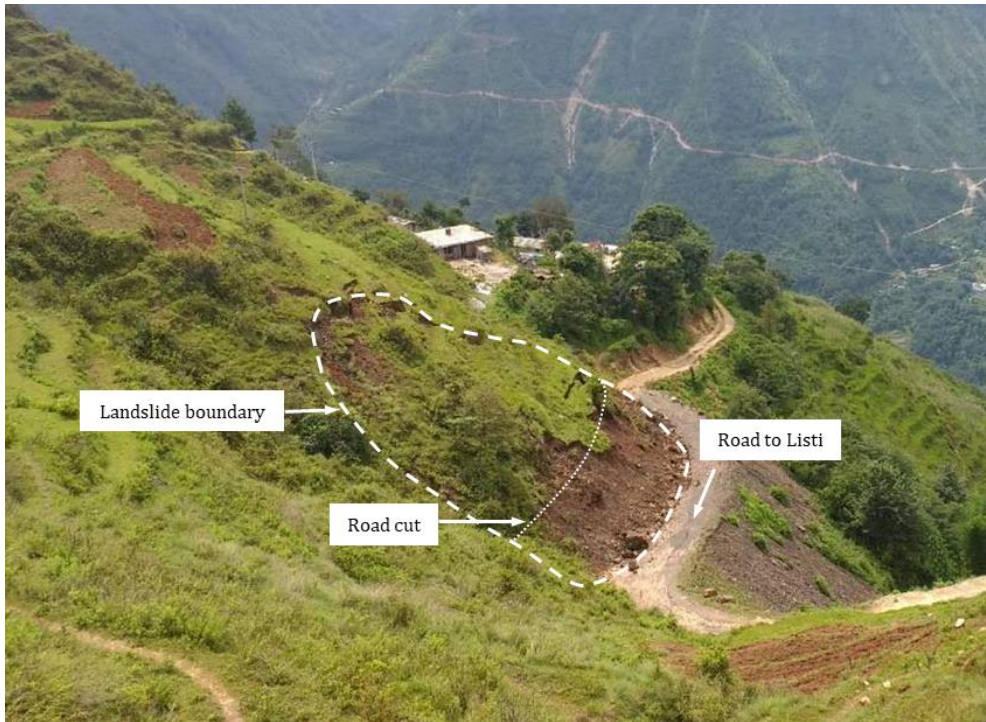
Figure 2.16 Failure in cut slope extending to hillslope (27°53'8.20"N 85°52'45.30"E).
