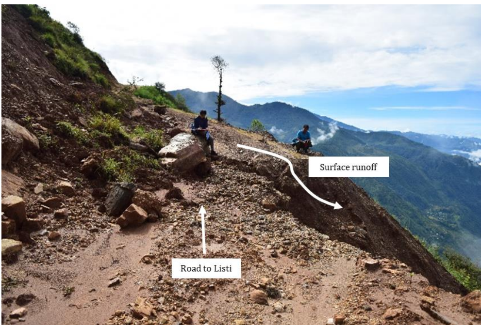
Figure 2.19 Failure in original valley slope due to surface runoff (27°53'19.5"N 85°52'42.8"E).
