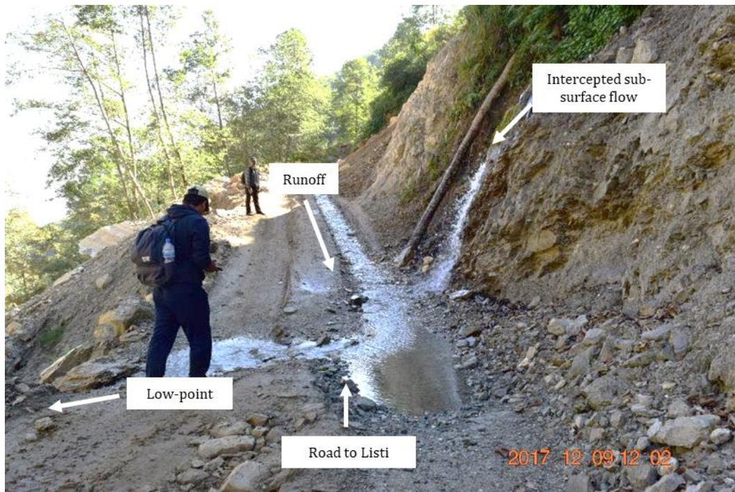
Figure 2.11 Improper surface and subsurface flow management along Daklang-Listi road ( 27^{\circ}53'24.3''\text{N} 85^{\circ}53'18.5''\text{E} ).
