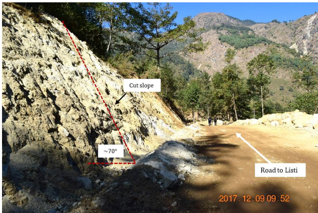
Figure 3.1 Road-cut slope at Kanglang landslide before failure (December 2017) (27°53'32.0"N, 85°54'28.5"E).
