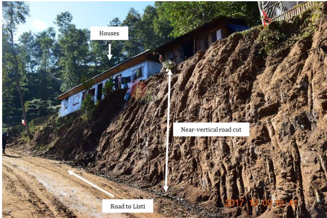
Figure 2.7 Steep road-cut slope adjacent to the settlement area along Daklang-Listi road ( 27^{\circ}53'30.0''\text{N} 85^{\circ}54'09.2''\text{E} ).
