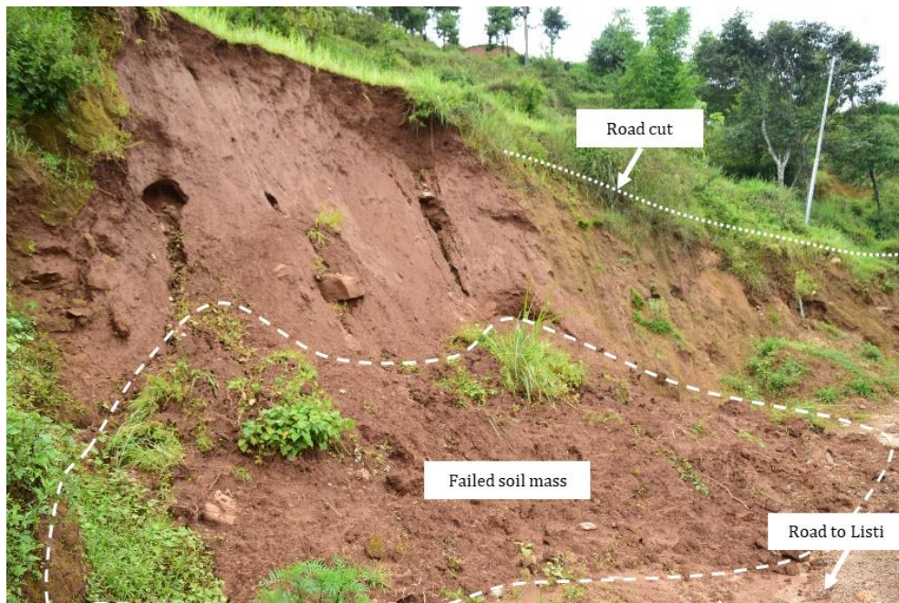
Figure 2.17 Failure in cut slope only (27°53'06.5"N 85°52'47.2"E).
