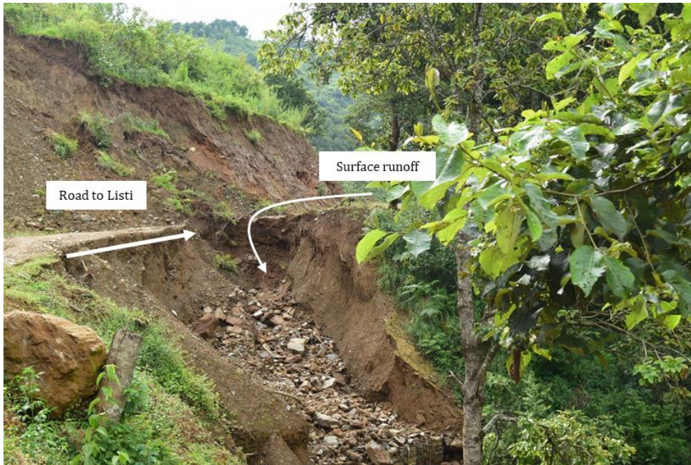
Figure 2.18 Failure in original valley slope due to surface runoff (27°53'11.70"N 85°53'28.10"E).
