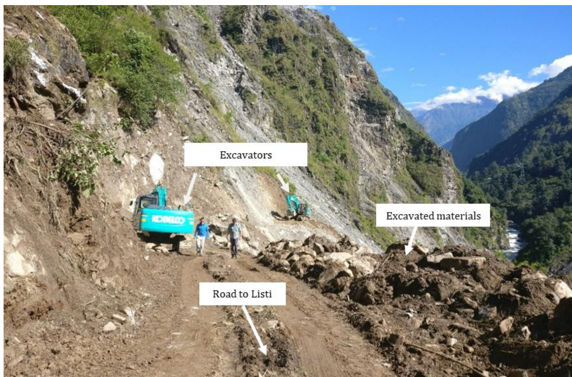
Figure 2.5 Construction of Daklang-Listi road, looking North ( 27^{\circ}53'49.20''\text{N} , 85^{\circ}54'46.20''\text{E} ) (*photo location shown in Figure 2.6).
