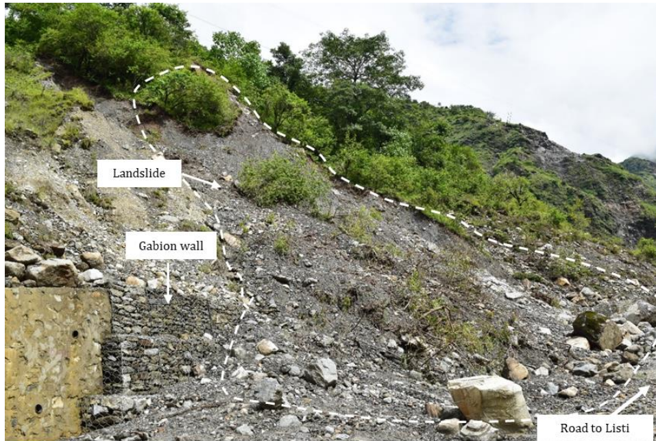
Figure 2.22 Gabion wall overtopped by landslide debris (27°53'43.2"N 85°54'48.0"E).
