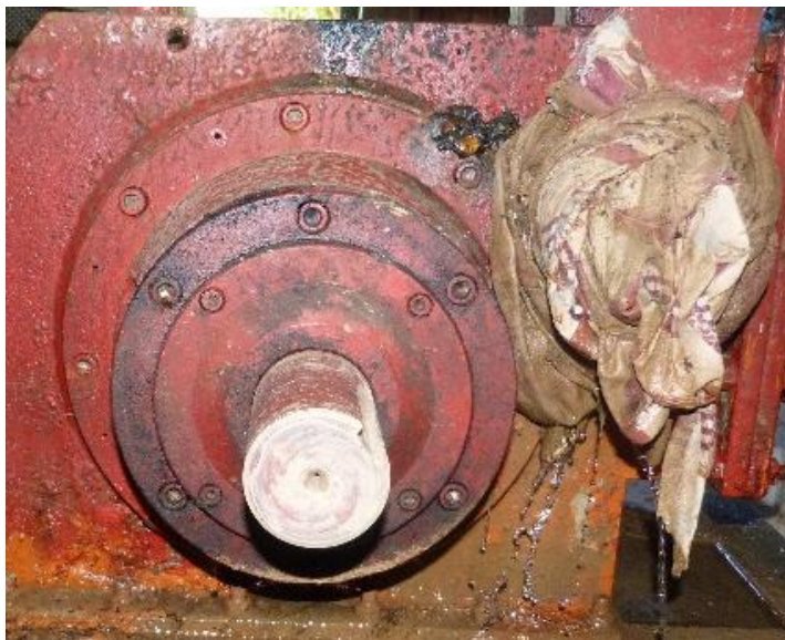
Figure 4.4 - Leakage from a turbine casing. Photo credit, author.
