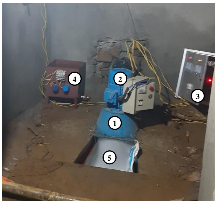
Figure 7.18 - Turbine-generator set, ballast tank and control panel inside the powerhouse. Numbered labels indicate: 1 – turbine casing, 2 – generator, 3 – control panel including ELC, 4 – ballast tank, and 5 – tailrace. Photo credit, Prem Karki.
