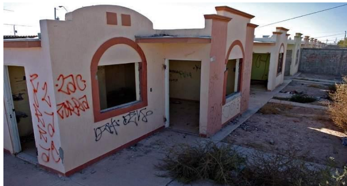
Figure 1. Abandoned social housing in Tijuana. (Notimex, 2019)
