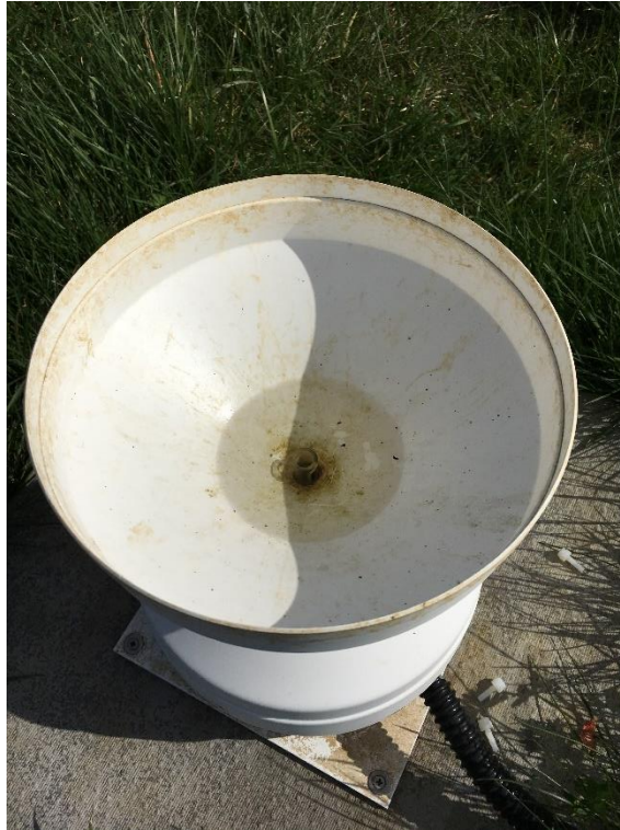
Figure 2-6 Example of a blocked TBR (Source: Personal collection).
