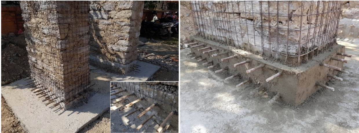
Figure 8 Wire mesh tied and welded to the rebar of the pedestal (left); Connections covered with 50mm of 1:6 plaster (right)
