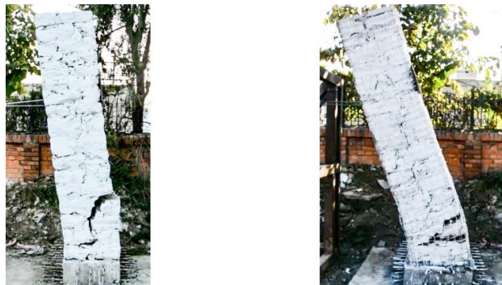
Figure 11 Final deflected shape of the unretrofitted (left) and retrofitted (right) wall before collapse
