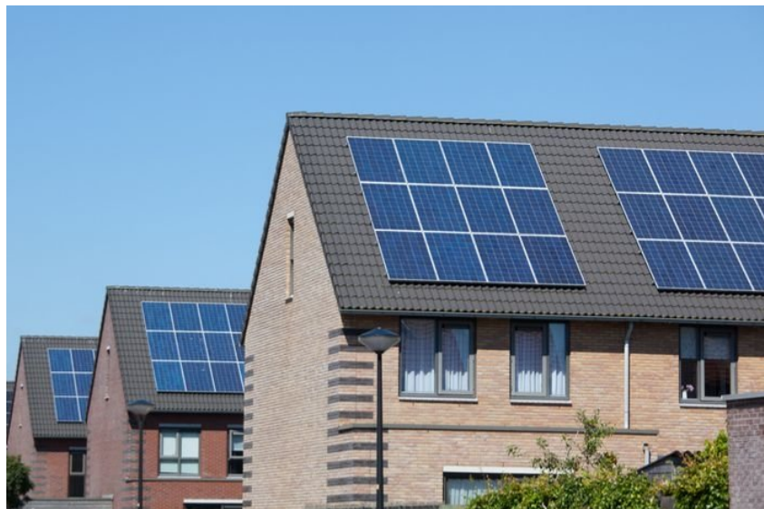
Figure 2-1 Rooftop Photovoltaic Panel
