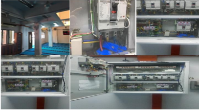
Figure 3: Installation of our energy monitoring system.
