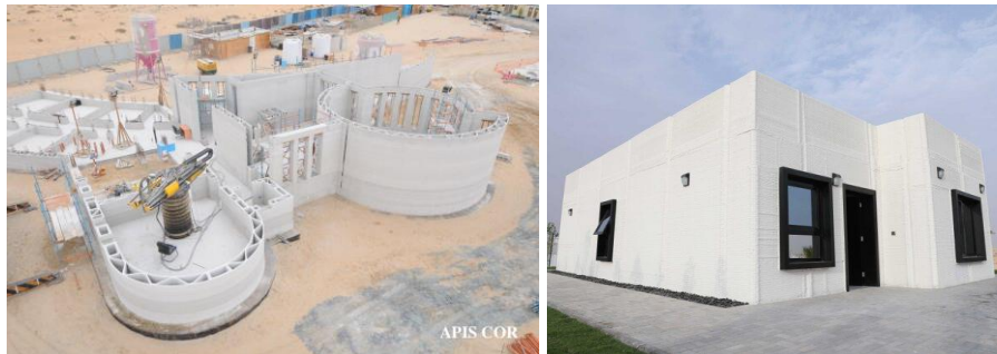
65 66 Figure 1: Notable examples of 3DP concrete buildings: (a) Two-storey office building in Dubai 67 constructed by Apis Cor (image credit: Apis Cor), and (b) House in Saudi Arabia constructed by 68 CyBe (image credit: CyBe).
