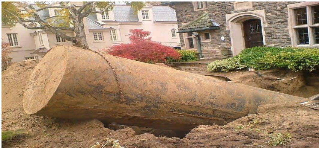
Figure 3:3 Obstruction hazard example of an old oil tank found underground
