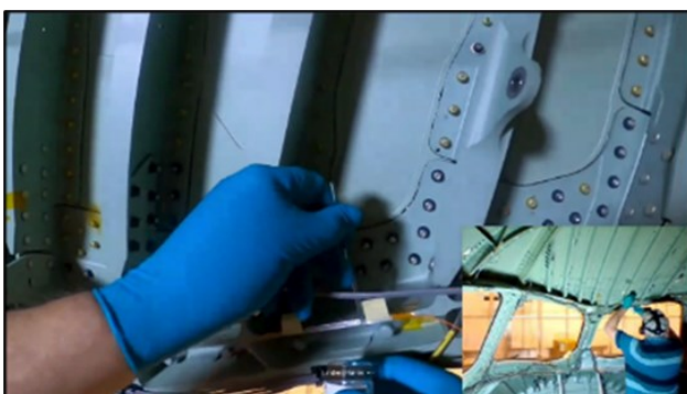
Figure 7. Installation of DIMES sensors by the Topic Manager on an aircraft fuselage at Airbus, Toulouse, with remote support from the DIMES partners.
