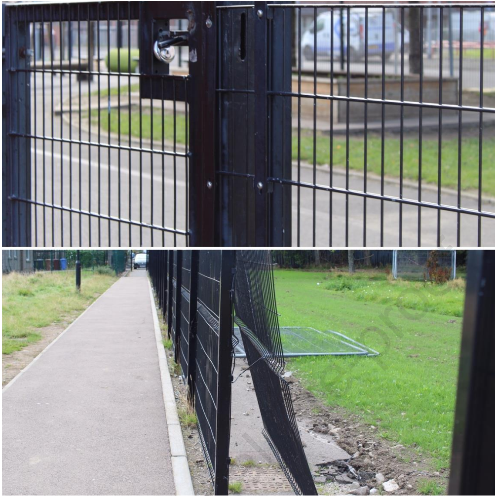
Figure 2a Secure fence around school Figure 2b Broken fence around school
