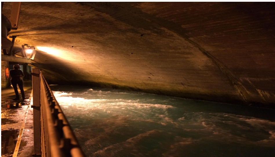
Inside the hydroelectric power plant
