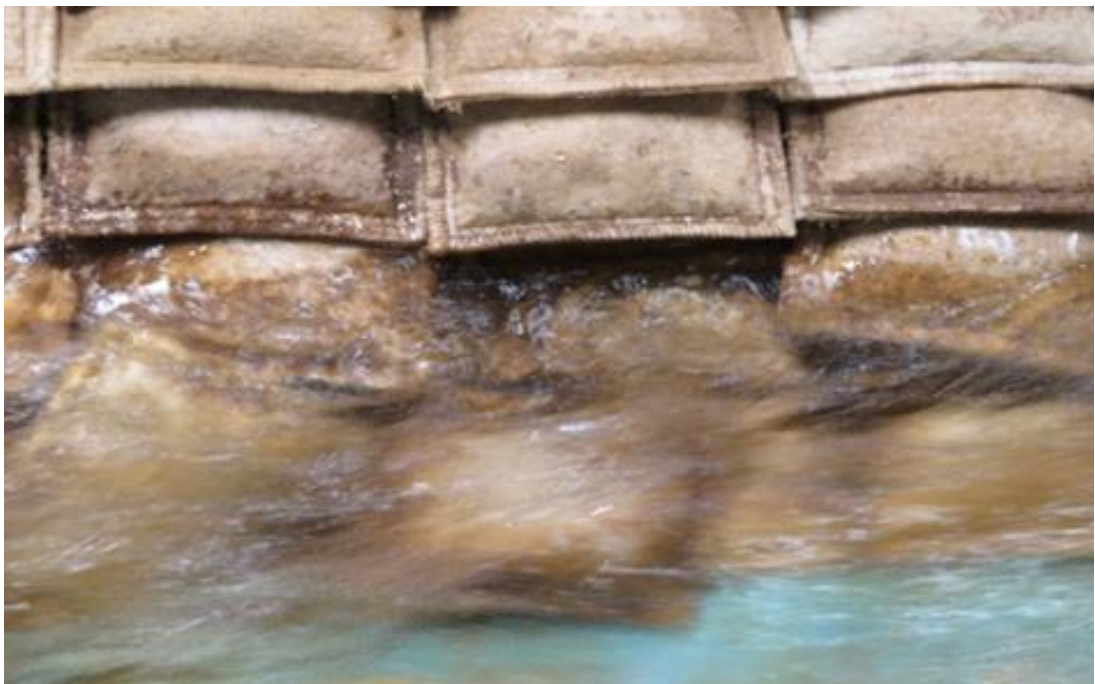
(a) Initial displacement due to turbulent bursting–induced flow through revetment voids and sliding, low water level
