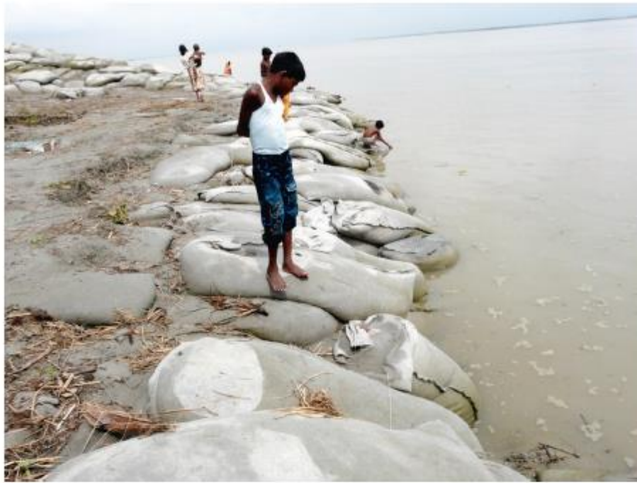
(c 1) Inadequate thickness of geobag revetment
