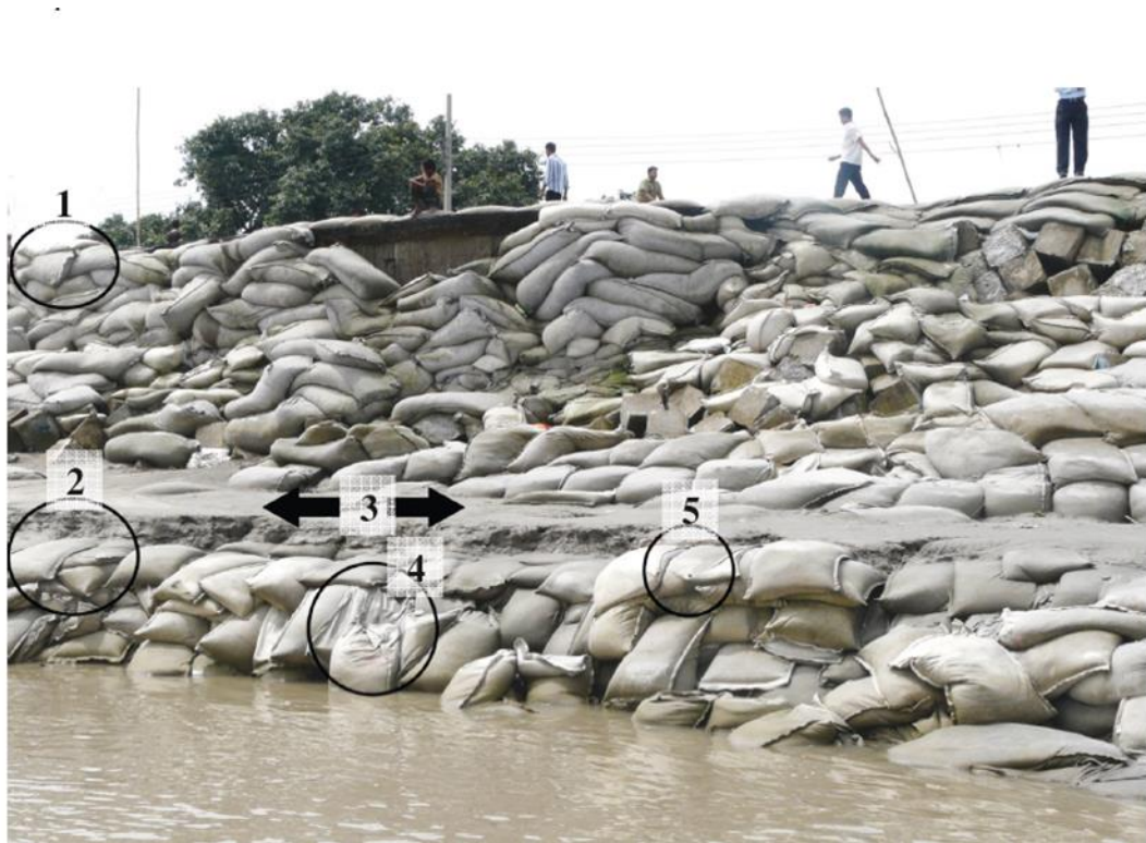
Figure 2.8: Failure modes in geobag revetment (JMREM, 2006; Akter, 2011): 1: Pullout; 2: Slump; 3: Dislodgement of the top bag; 4: Slide; 5: Physically damaged
