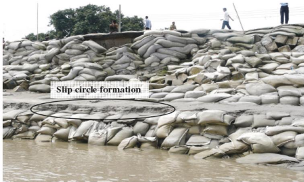
(a 1) Displacement due to rapid drawdown
