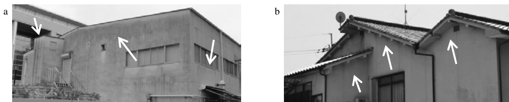
Fig. 3. (a) Walls directly exposed to rainwater; (b) walls rarely receiving rainwater.
