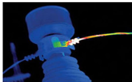
Fig.1.7: Identifying unexpected heat loss in electrical connections
